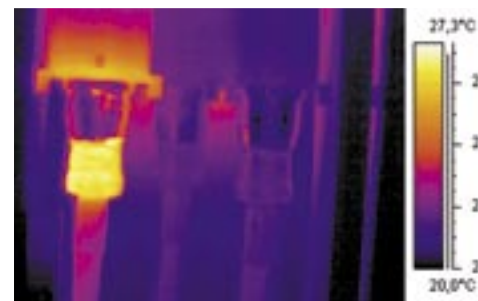
To decide whether a hot-spot is a real problem or not, you need to be acquainted with the installation.
