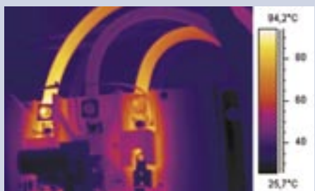
Poor connection and internal damage
